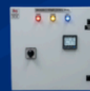
EMERGENCY PUSH BUTTON
