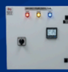
EMERGENCY PUSH BUTTON
